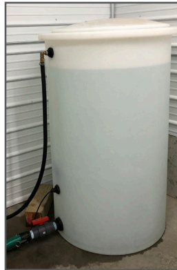
250-gallon holding tank, floats and supply plumbing
